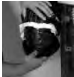
figure 7.2 Insert vinyl duct over the hooks and seal with a 30" tie wrap.
