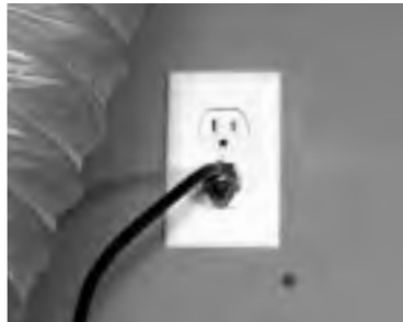
figure 9.2 Electric Wall Outlet
